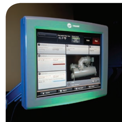
Tracer AdaptiView™ chiller controls
